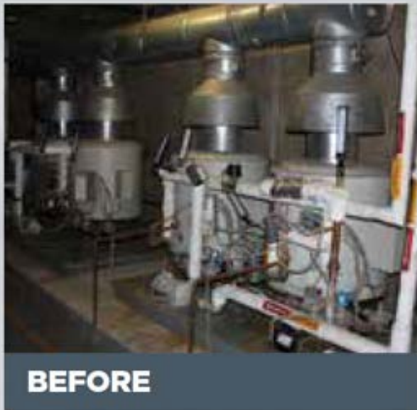
Domestic Steam Boiler
